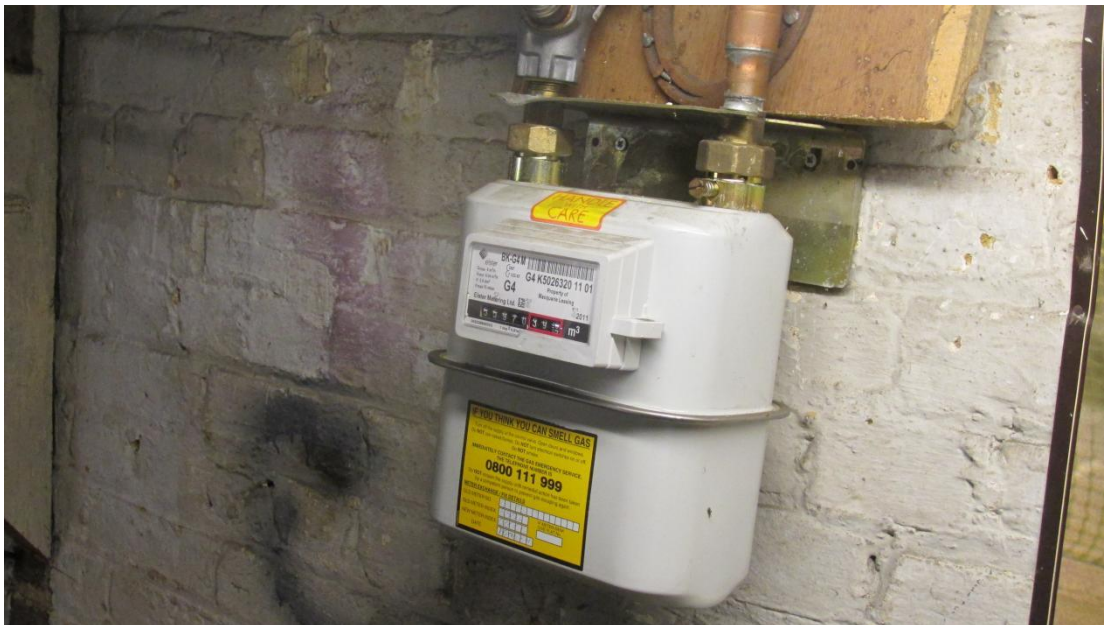
Gas meter in garage
