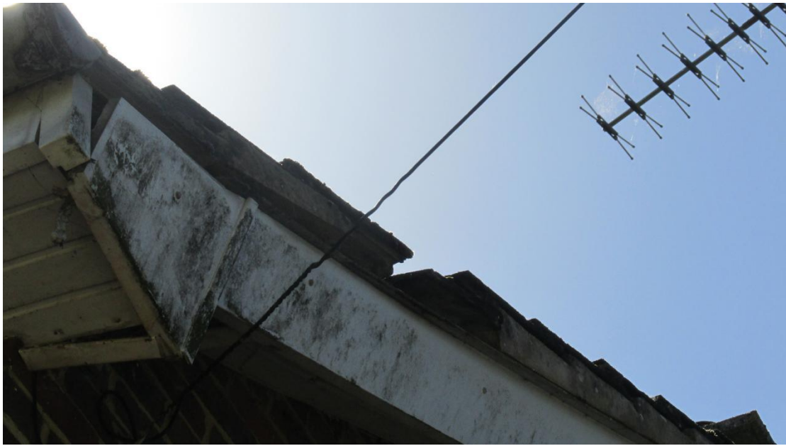
Broken soffits and barge board at the front right
