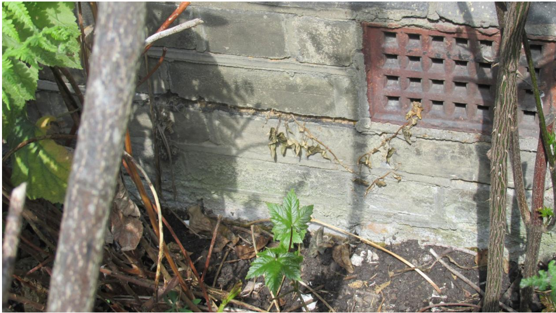
Wall under the bay window
