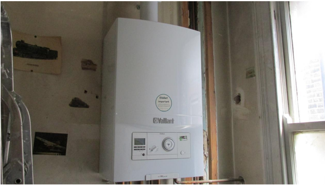
Boiler in the 1 st floor cupboard
