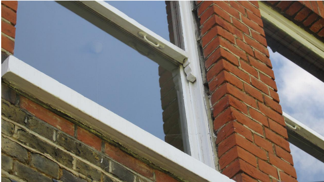
Missing pointing from the rear wall
