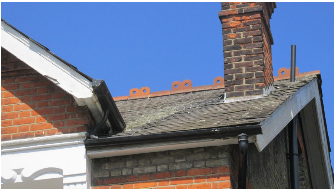
Soil vent pipe through the roof but bird protection cage is missing
