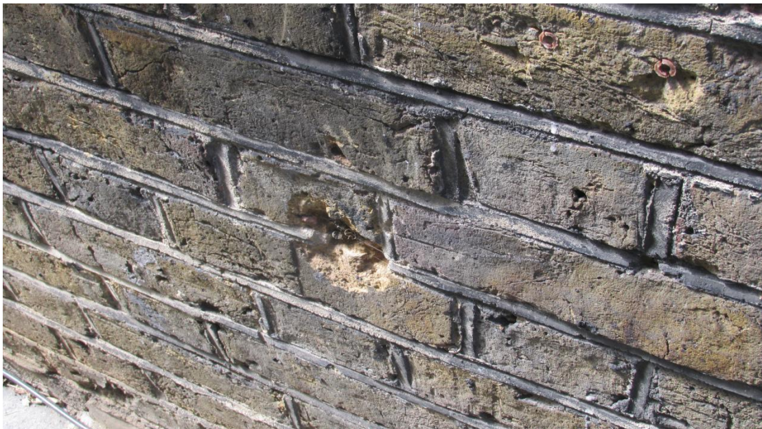
Damaged bricks on the side wall
