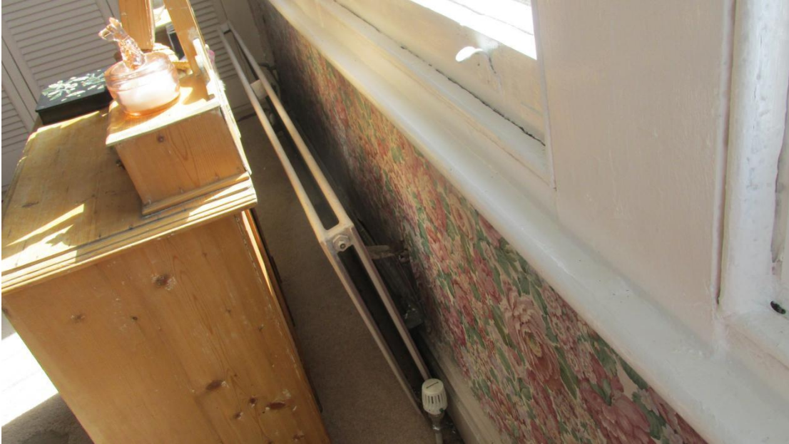
Radiator in the front bedroom
