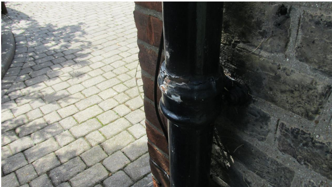
Damaged downpipe at the front
