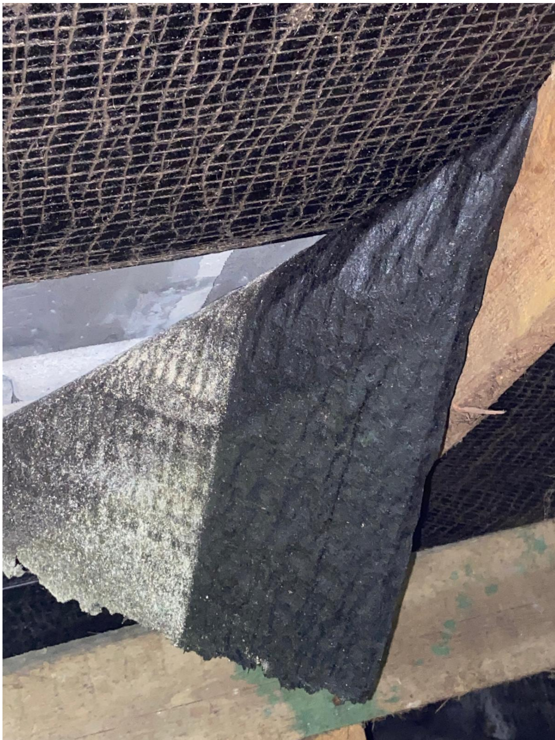
Broken felt under tiles
