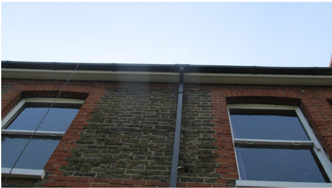
Gutters at the rear
