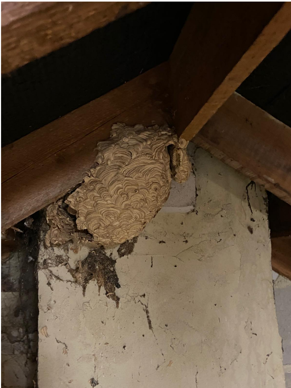
Wasp nest in the roof space
